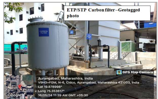
ETP / STP plants & carbon filters in MGM campus
